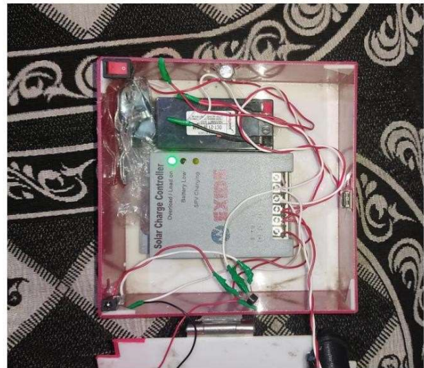
(Fig 3) Charge Controller
